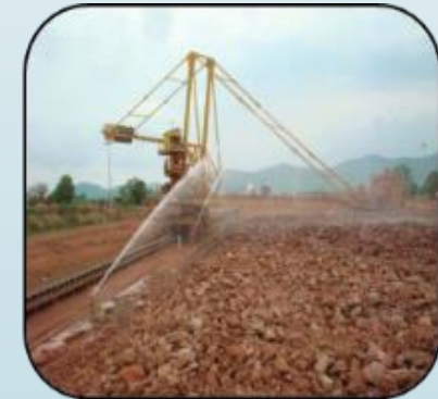
Water sprinklers at bauxite handling
