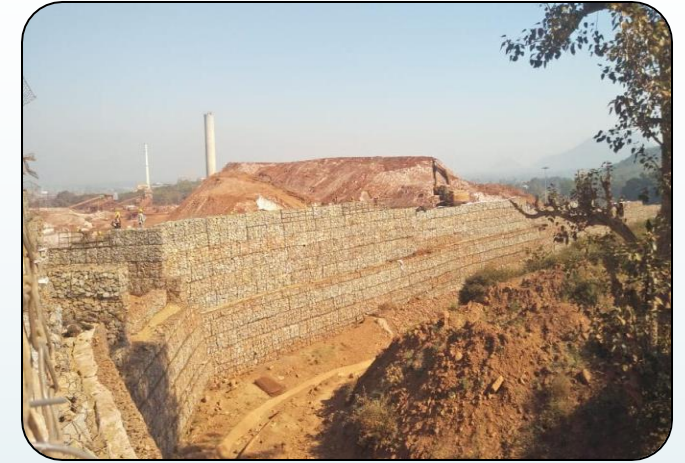
Gabian Wall installation for Life enhancement of existing pond by space augmentation
